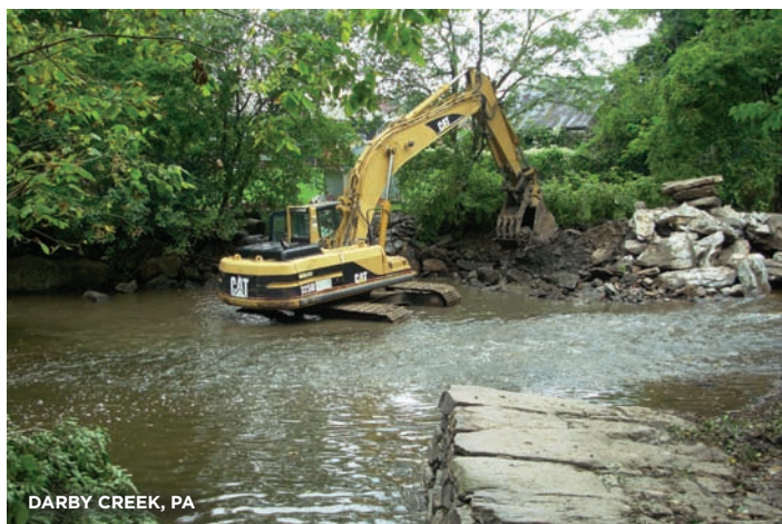
Just outside Philadelphia, we removed three dams, restoring 9.7 miles of Darby Creek, improving fish habitat, and reducing flood risk.
